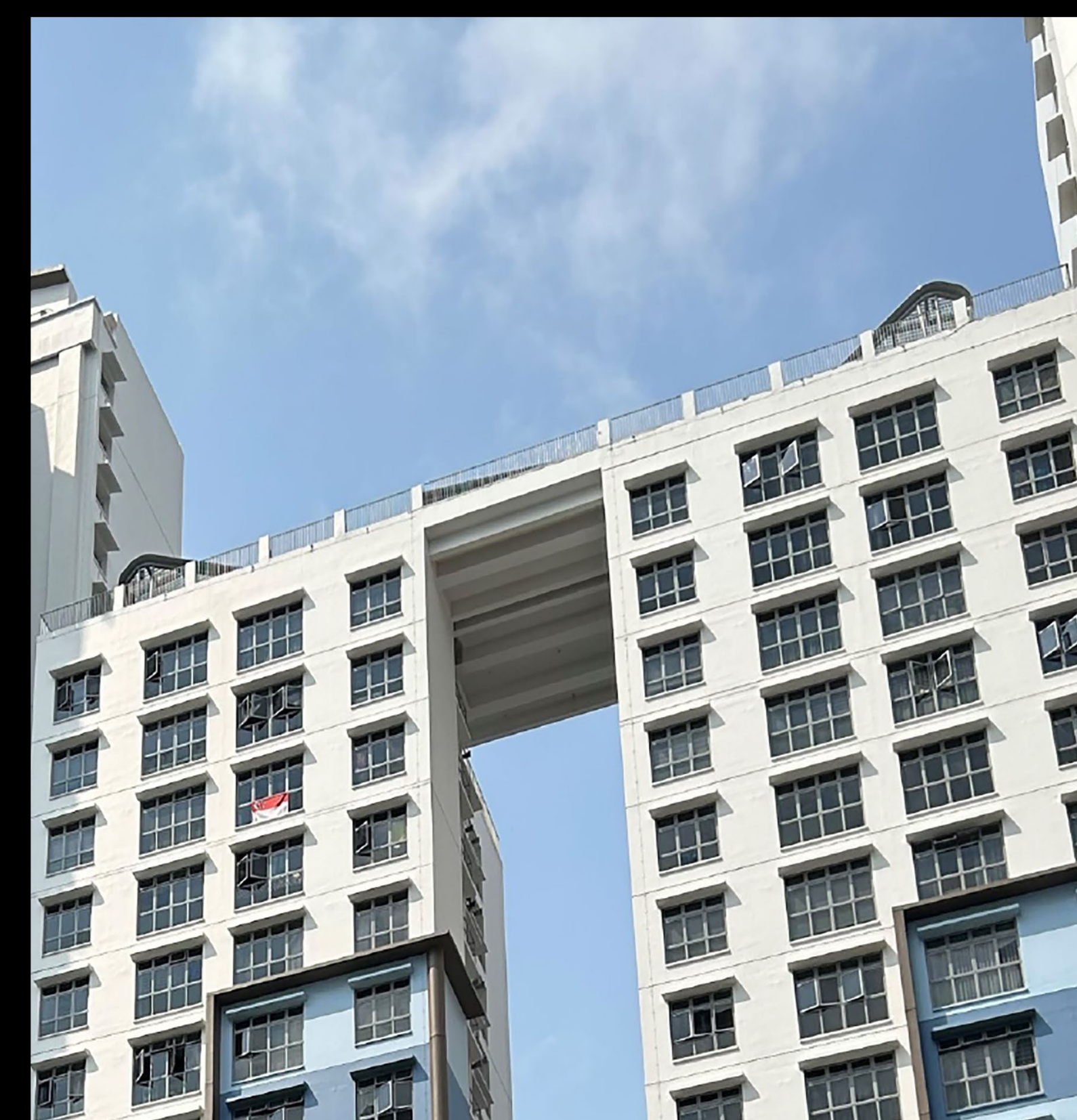
Link bridge at 19 th storey between Blocks 423A and 423B supported by precast N-profile beams
